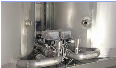
Continuous level measurement and motor ball valves
